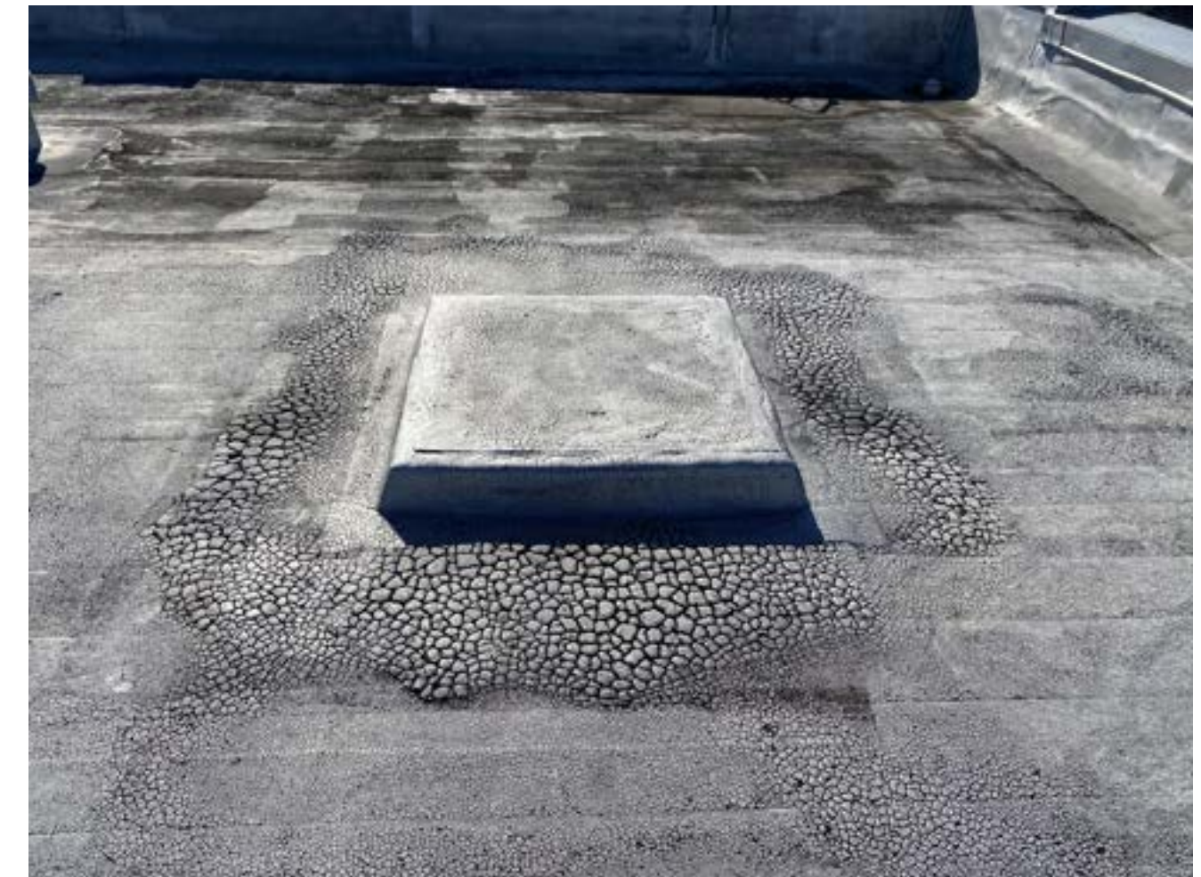
EXISTING ROOF - NEEDS REPLACEMENT.
