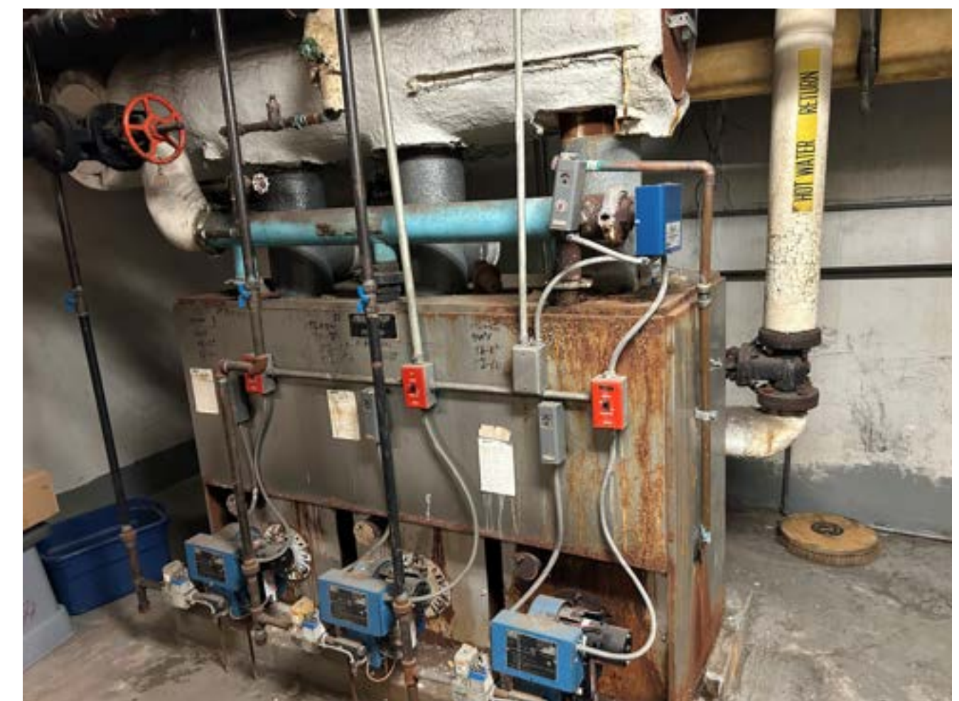
EXISTING MECHANICAL BOILER - NEEDS TO BE ABATED/REMOVED FOR OVERALL ENERGY CONSERVATION UPGRADE.
