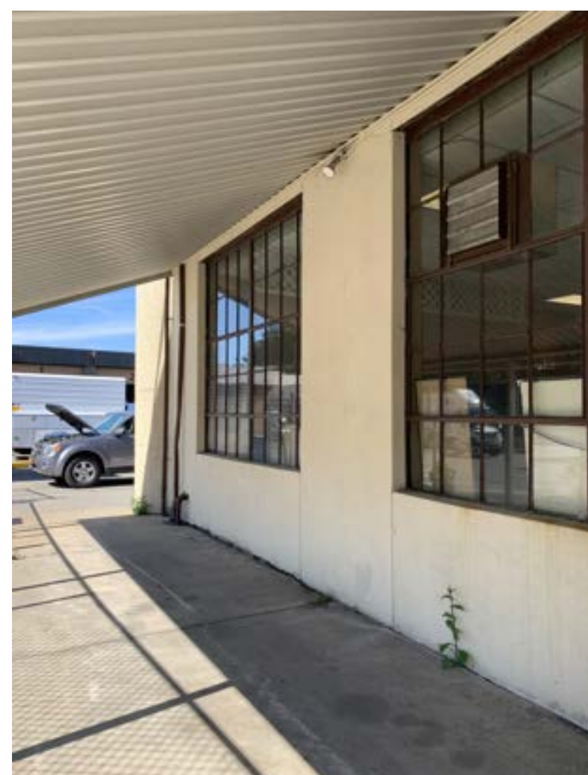
WINDOW REPLACEMENT - NEEDED FOR OVERALL ENERGY CONSERVATION UPGRADE.
