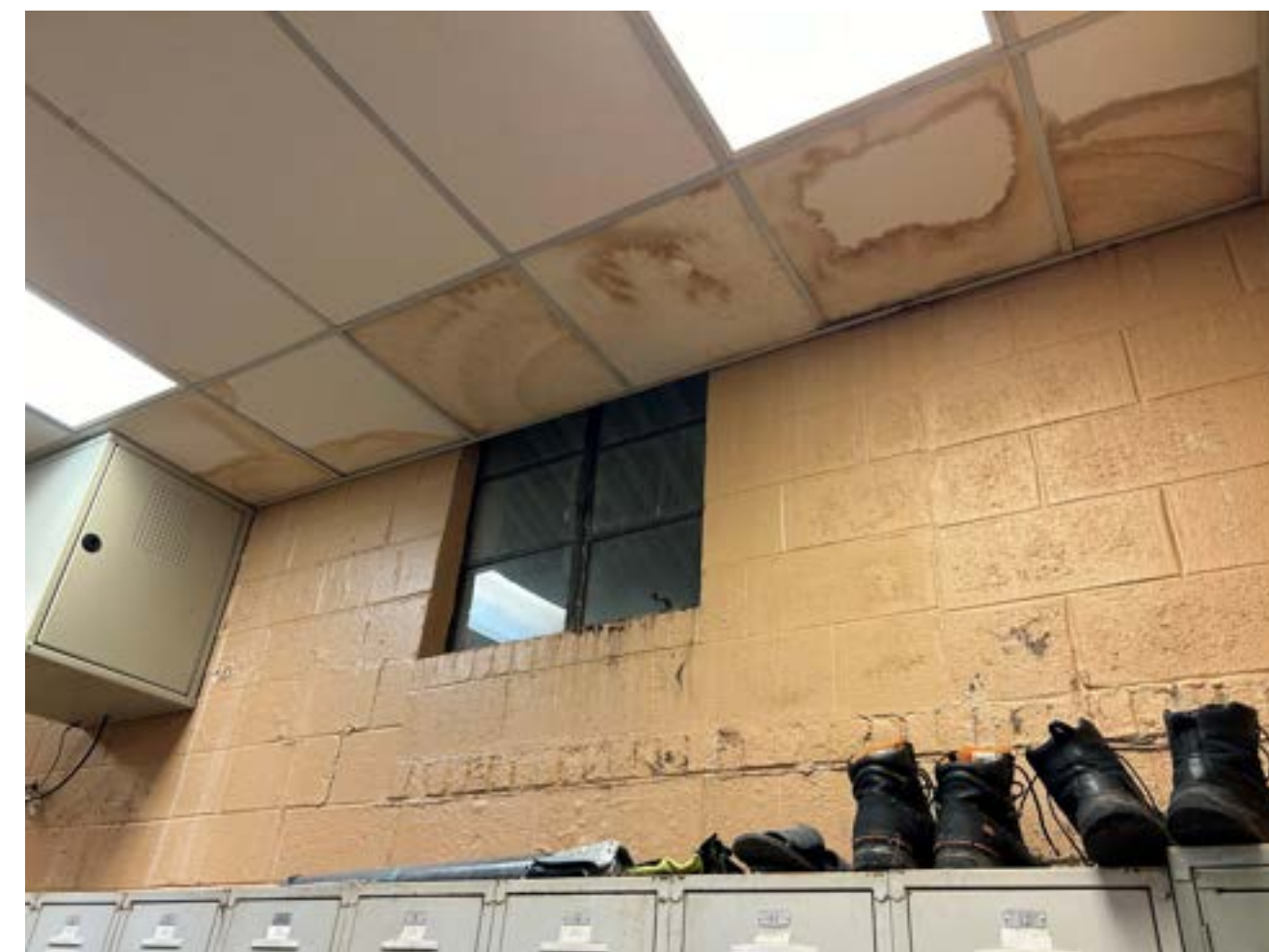
LOCKER ROOM - NEEDS REPAIRS/UPGRADES.
