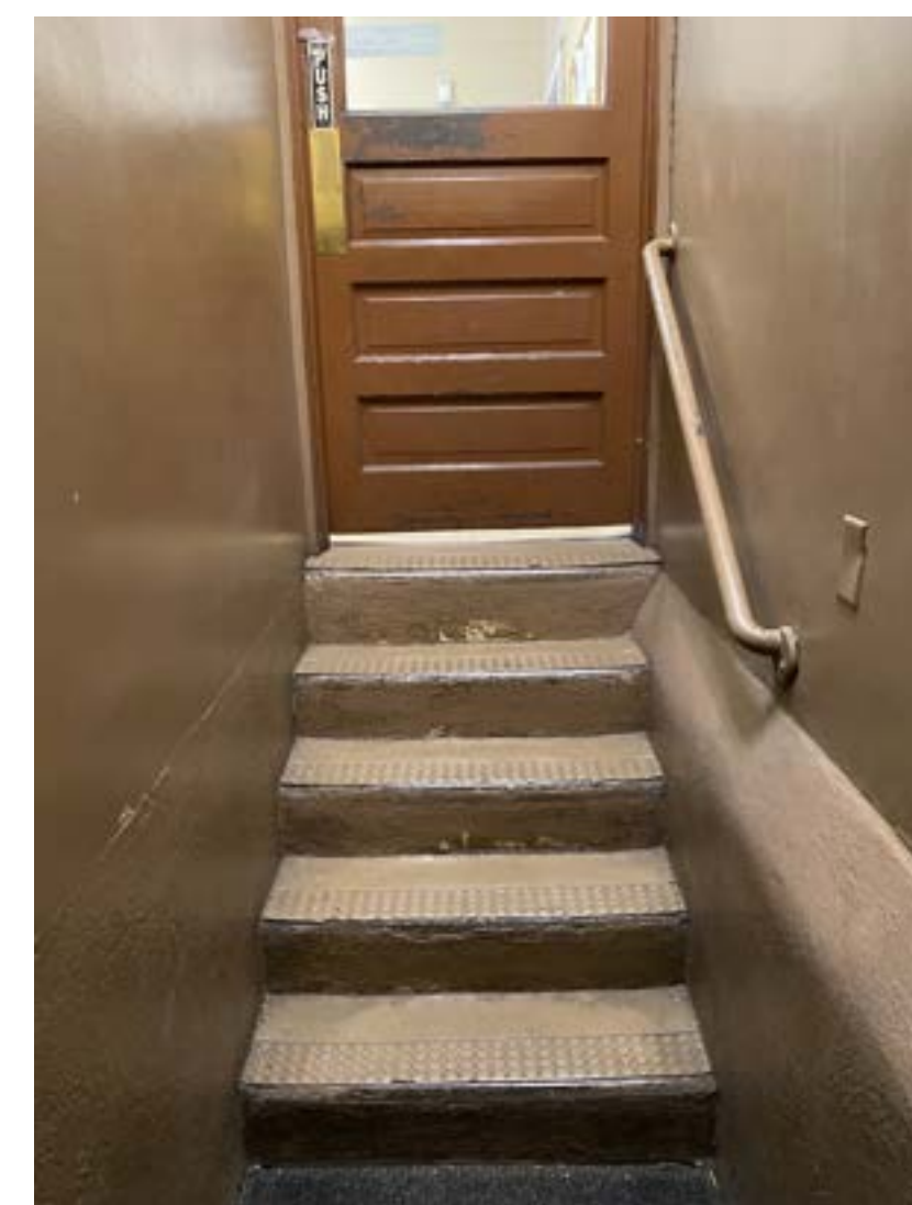
ACCESS TO OFFICE AREAS - NEEDS ADA HANDICAP ACCESS.
