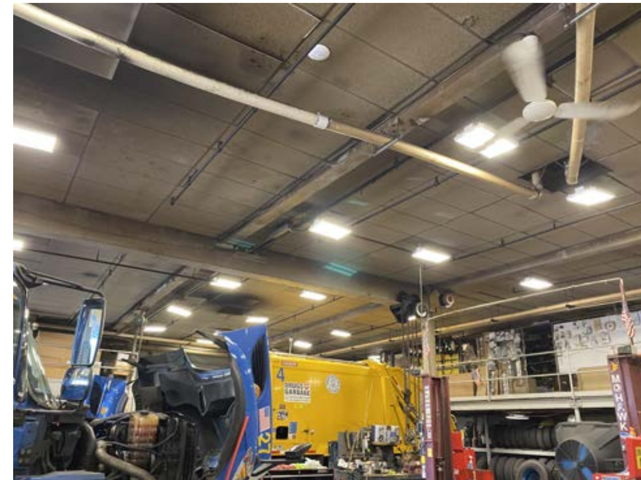
EXISTING MECHANICS GARAGE AREA - NEEDS REPAIRS/UPGRADES.
