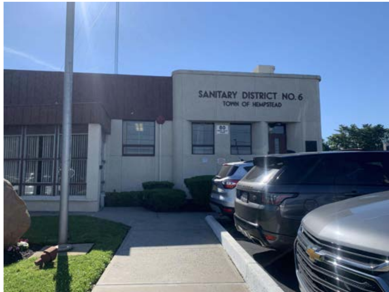
EXISTING FRONT ENTRANCE - NEEDS ADA HANDICAP ACCESS.
