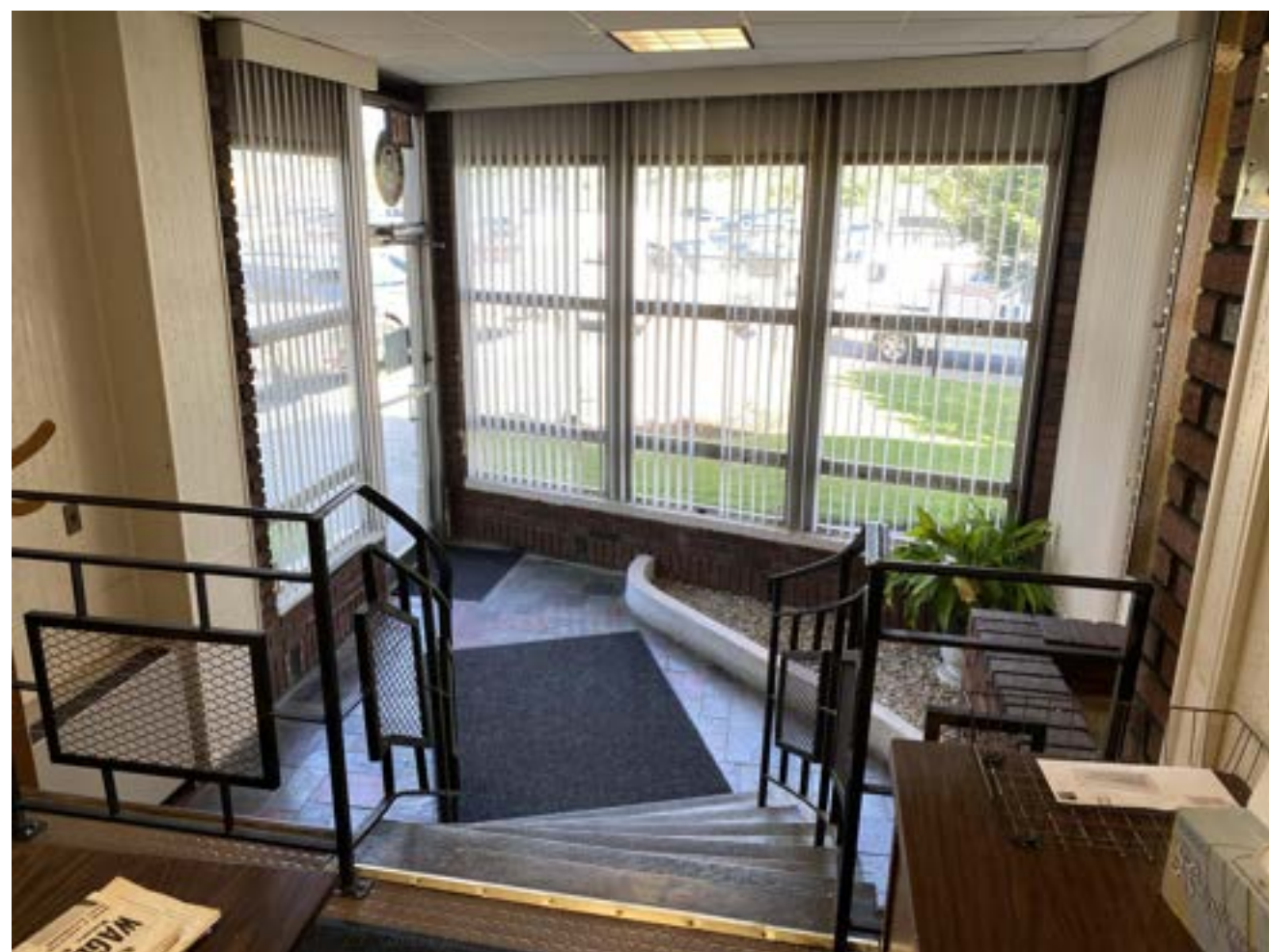
EXISTING INTERIOR FRONT ENTRANCE - NEEDS ADA HANDICAP ACCESS.
