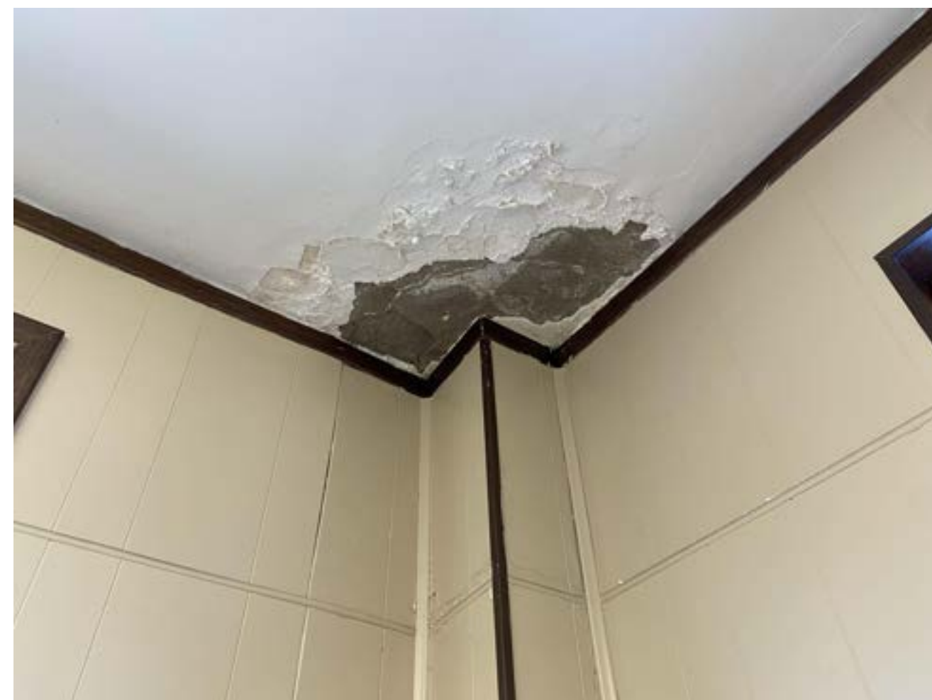
ROOF REPLACEMENT - NEEDED DUE TO LEAKS IN SEVERAL AREAS.
