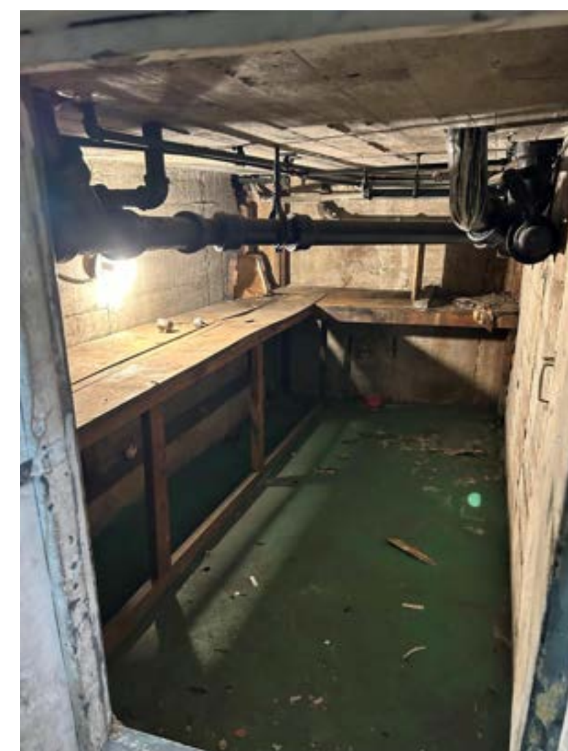
EXISTING CELLAR - HEIGHT ISSUES WITHIN USEABLE AREAS.
