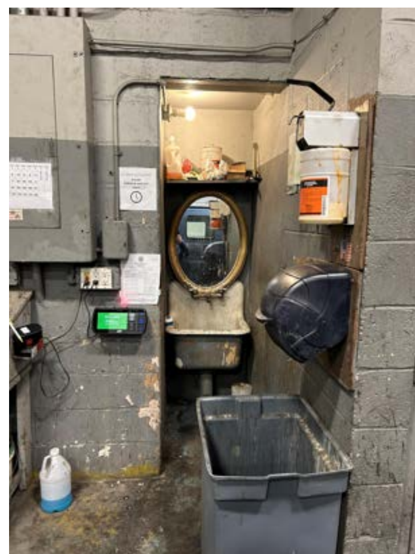
EXISTING MECHANICS GARAGE AREA - NEEDS REPAIRS/UPGRADES.
