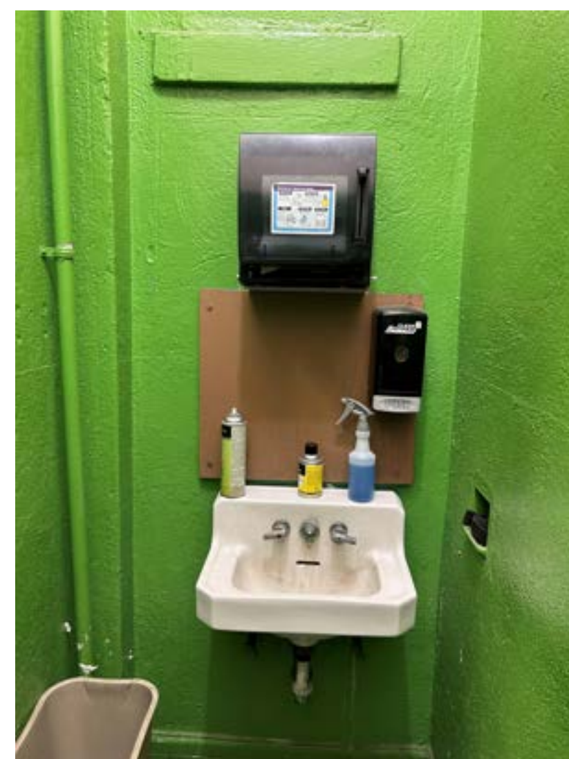
EXISTING RESTROOMS - NEED UPGRADES AND ADA HANDICAP ACCESS.
