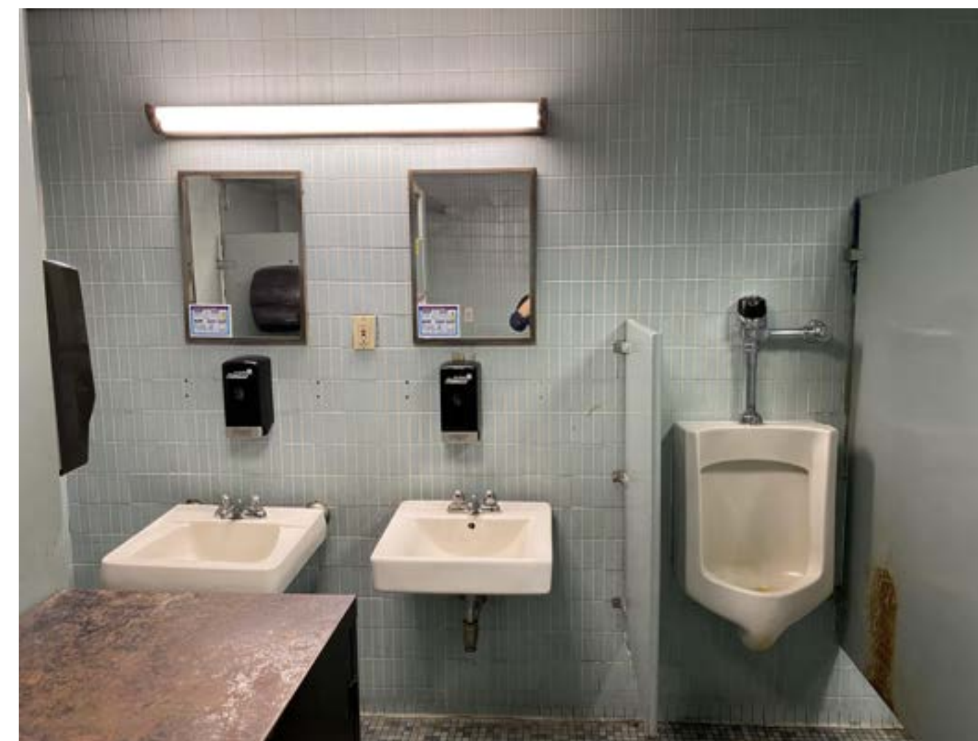
EXISTING RESTROOM - NEEDS REPAIRS/UPGRADES.
